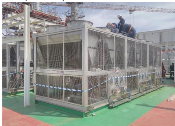
Fig. 2. HVAC (Air Cooled Chiller) Unit
