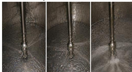
Fig. 5 Water Pressure Instability
