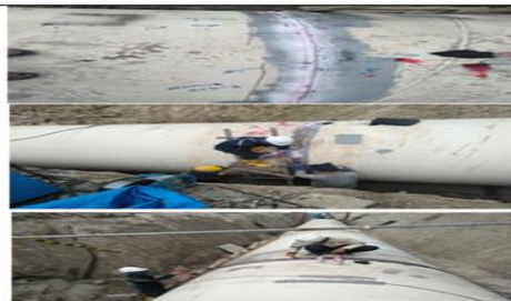
Fig 4, 5 and 6. Photo/Doc of NDT-PT welding testing Source: Doc/Photo QA/QC Mechanical PLTM Parmonangan The findings in the field were that the welding results of the Water Way and Penstock pipes met the Rejection Criteria, welding defects were found, for this reason repair work/repeated welding work was carried out again.
