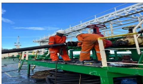
Fig. 4. Bunker hose flange leak Source: Researcher Documentation (2025)
