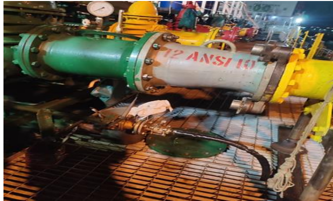
Fig. 4. Indications of a leak
