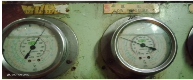
Fig 1. High and low pressure manometer
