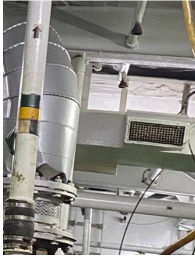
Fig 8. Blower In and Blower Out
