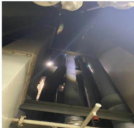
Fig 3. Exhaust Gas Entry into the Engine Room
