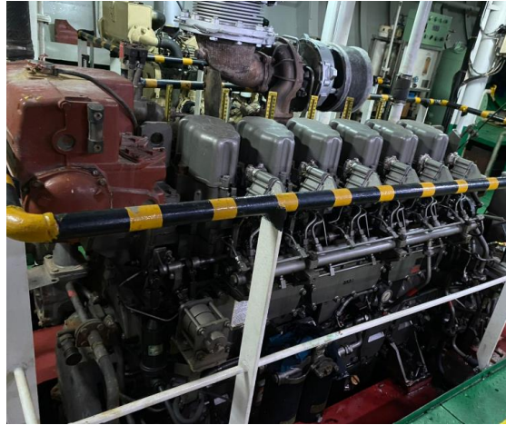
Fig 5. Engine Activity Increases Engine Room Temperature
